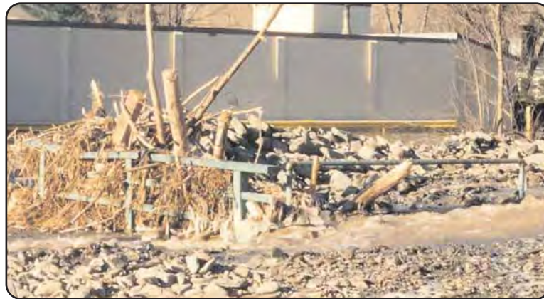
The bridge over the Bull Run on lower Main Street, Margaretville, clogged with debris in 1996. Photo courtesy Robert Halpern
