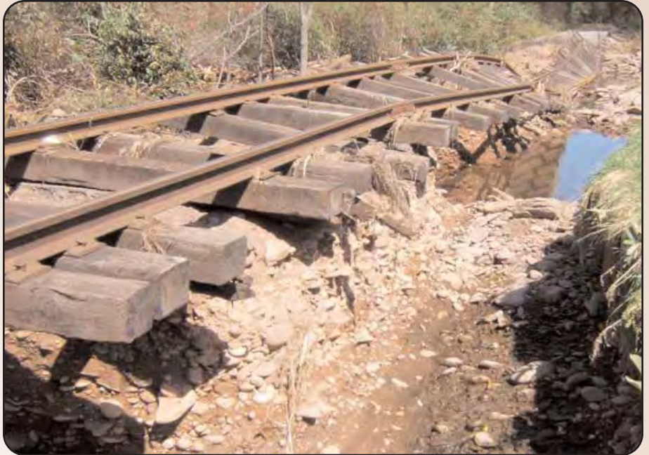
The Delaware & Ulster Railroad was forced to cut short its tourist excursion season this year when hundreds of feet of track, like this section in Kelly Corners, were washed out.
